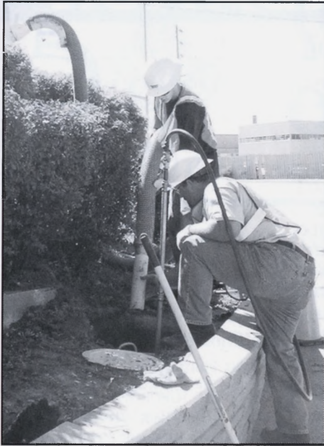
SUE Technicians installing a test hole at the intersection of Airport Road and Derry Road in Mississauga, Ontario.
